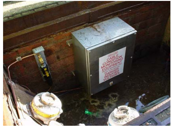
View of Pressure Transducer in Cable Pit
