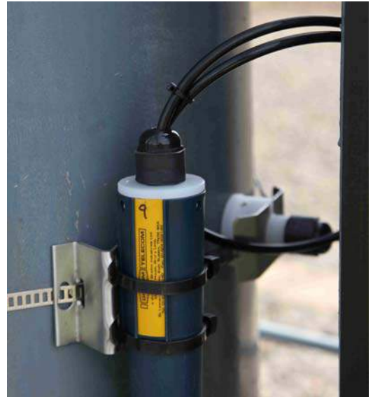
View of Temperature Transducer attached to oil expulsion tank
